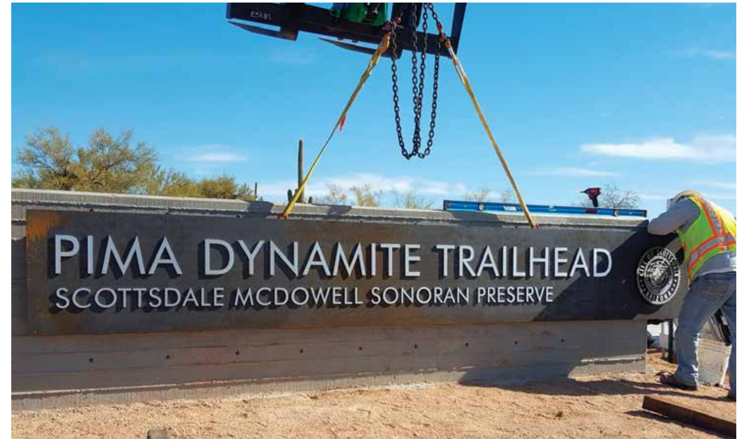
Crews install the monument sign at the Pima Dynamite Trailhead. Photo courtesy of City of Scottsdale.
